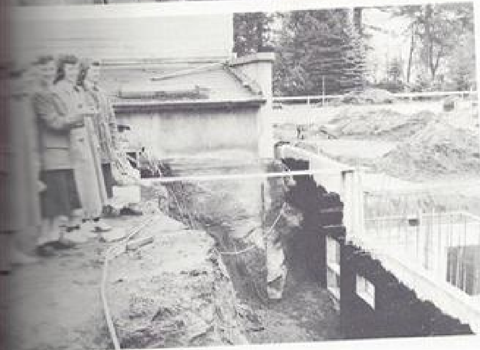
Alice Wayne, Peggy Webb, Kathy Leahy and Janice Carlson are taking quite an interest in - of all things - the new boiler room.
