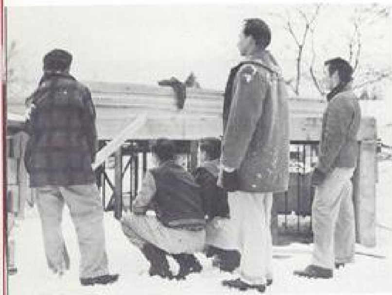
Sidewalk superintendents George Orr, David Kryger, Rodney Newby, Larry Anderson and Terry Semanko check building progress.
